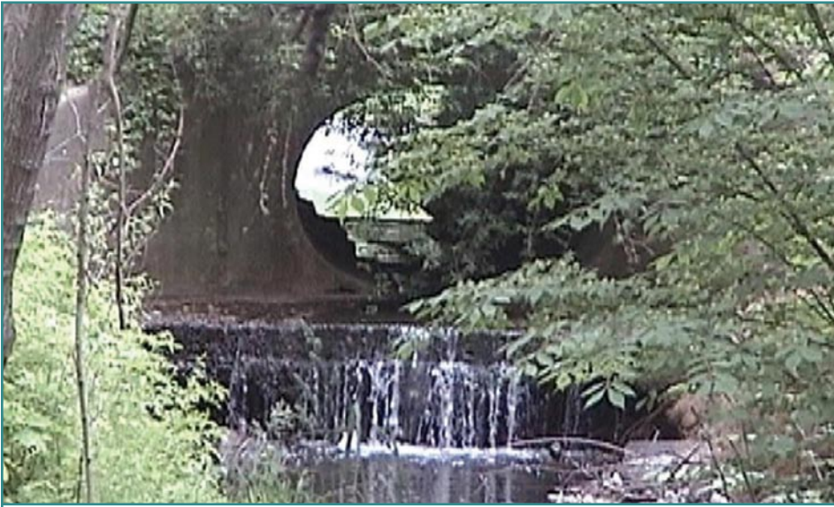
Erosion at the downstream end of a culvert creates a drop-off (waterfall), blocking fish passage.
